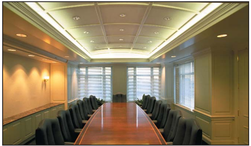
These coves are illuminated using a continuous row of model CLS fixtures, with Warm White (30TC) lamps.
